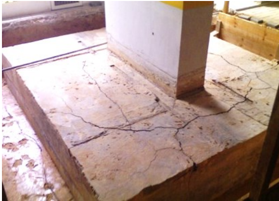
Figure 7 - Concrete foundation cracked due to DEF phenomenon
