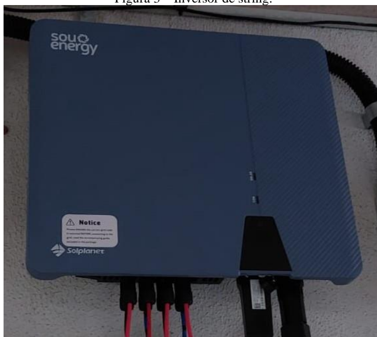
Figura 3 – Inversor de string.
