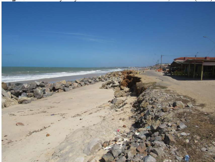
Fig. 10 Road destroyed by shoreline erosion on Icaraí beach, Caucaia (2019)
