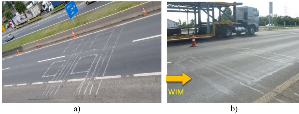
Figure 6. Final appearance of HS-WIM system in both highways: a) BR-381 [15]; b) BR-290 [16].
