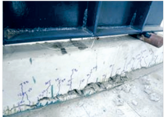
D VA-4 beam in the collapse
