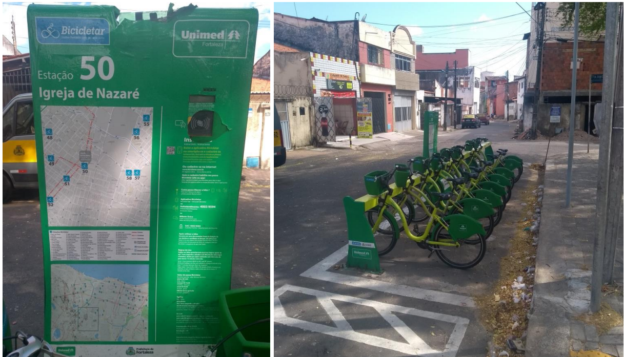
Totem damaged at the top / View of the station installed on the side of the street, next to the square
