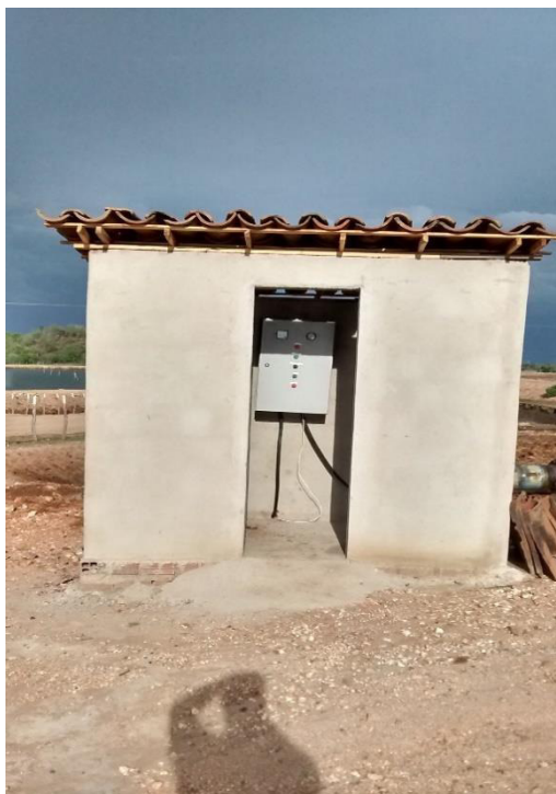
Figura 4 – Sistema soft start que protege as motobombas
