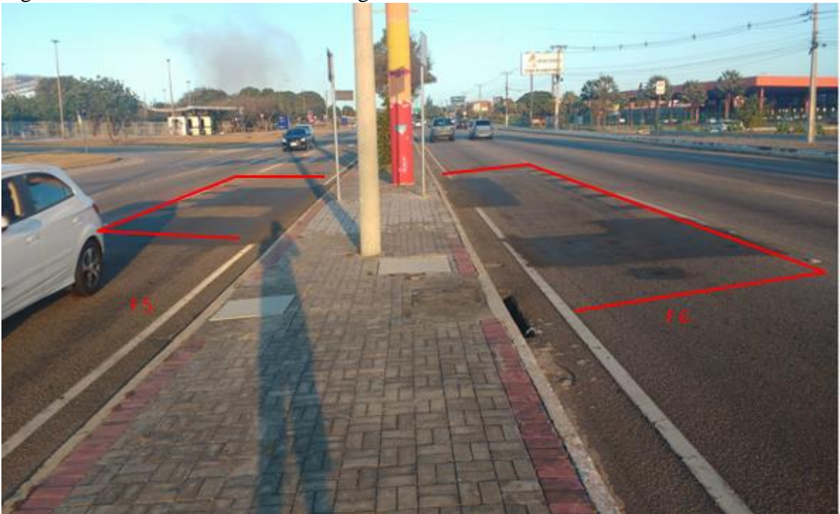
Figura 34 – Remendos devido as sondagens
