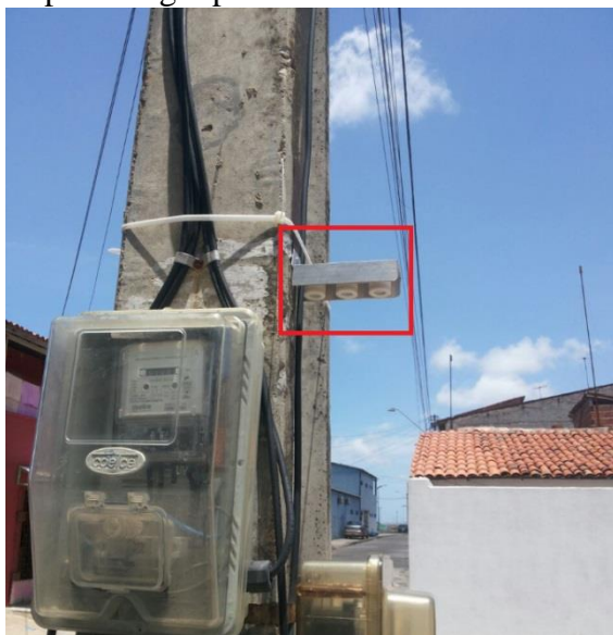
Figure 36 - Installed NO 2 passive sampler in public light post
