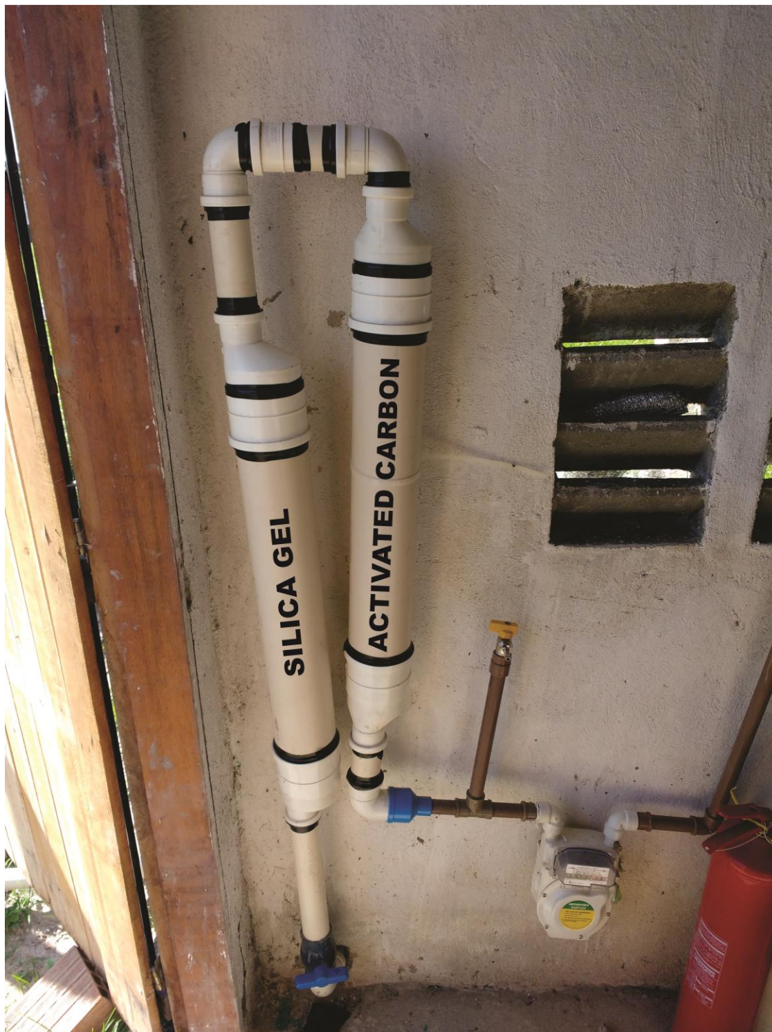
Figure 14 – Silica Gel and Activated Carbon Filters
