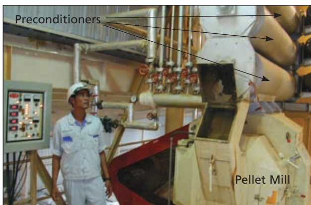
Multiple preconditioners are positioned above this pellet mill to moisten and heat meal with steam before it reaches the pellet mill.
