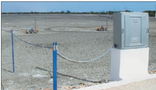
This growout pond is ready to be filled with water. Note the electrical cables connected to a control panel, with poles and aerators properly positioned.
