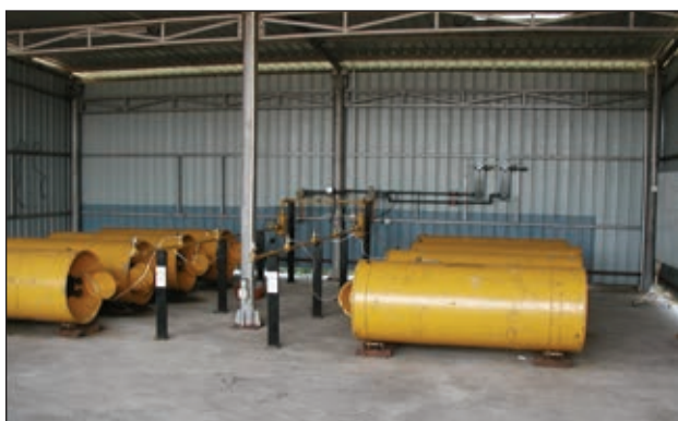
Gas chlorine cylinders controlled by flow meters treat pond inlet water.
