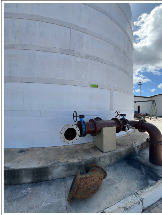
Figure 4 – Input flow into the homogenization and flow equalization tank
