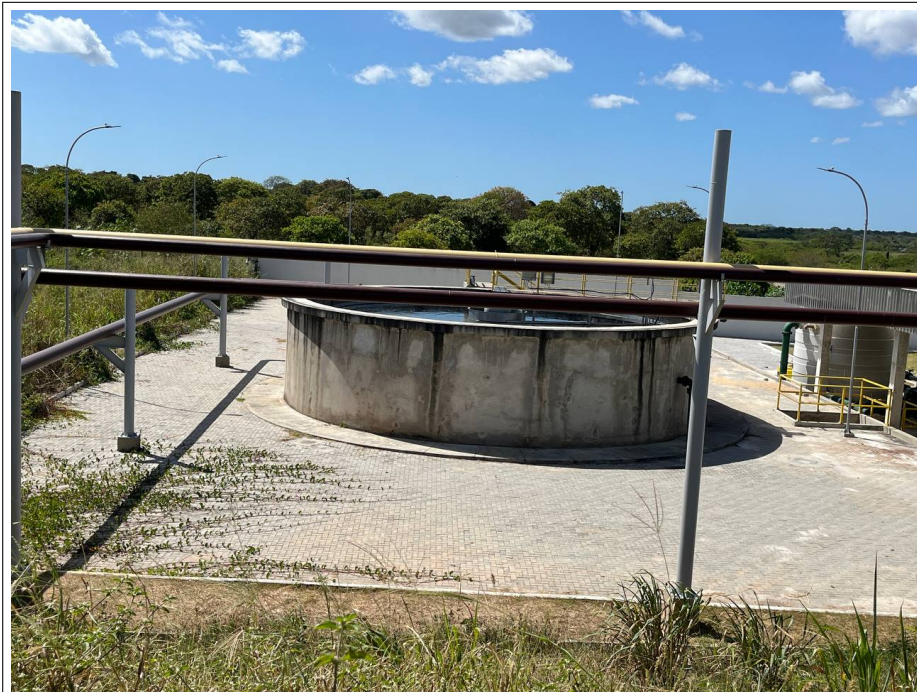
Figure 6 – Secondary settler at the analysed WWTP
