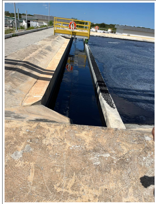
Figure 5 – Aeration tank during the process at the WWTP, filled with wastewater
