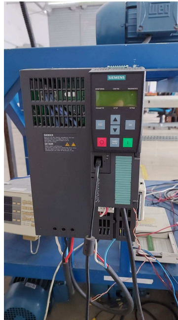
Figura 6 – Inversor Siemens - SINAMICS G120 PM250
