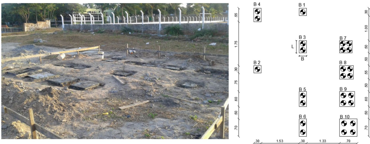
Fig. 2 a Photo and b schematic plan of the foundations analyzed (adapted from Cerqueira Junior 2019)
