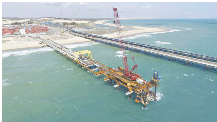
Figure 2. Aerial view of the Port of Pecém, showing the construction of a new bridge to access the berths piers.
