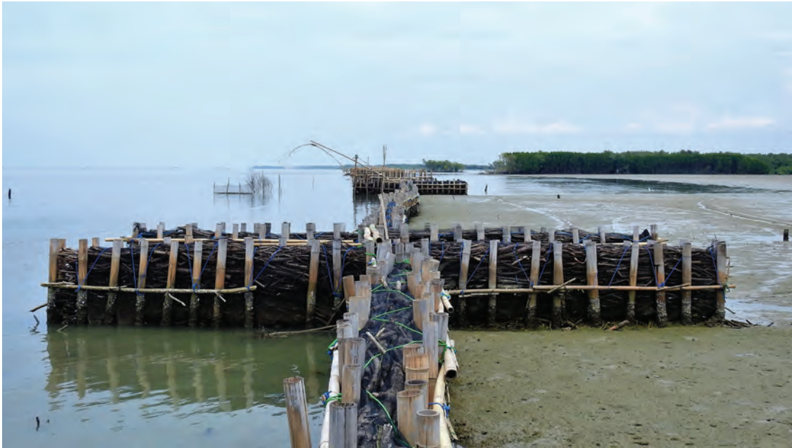
Holey wall: The aim of this porous sediment trap built by the Building with Nature Project in Demak, Indonesia, is to create suitable habitat for natural mangrove regeneration. Photo: Yus Rusila Noor
