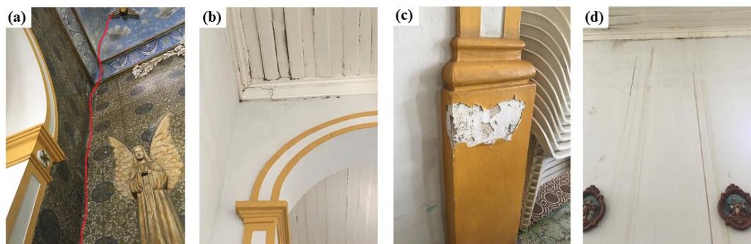
Figure 5. Internal pathological manifestations of the Nossa Senhora do Rosário Church: (a) crack, (b) disintegration of lining elements, (c) detachment and (d) humidity stains.
