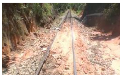
(a) Lastro colmatado
